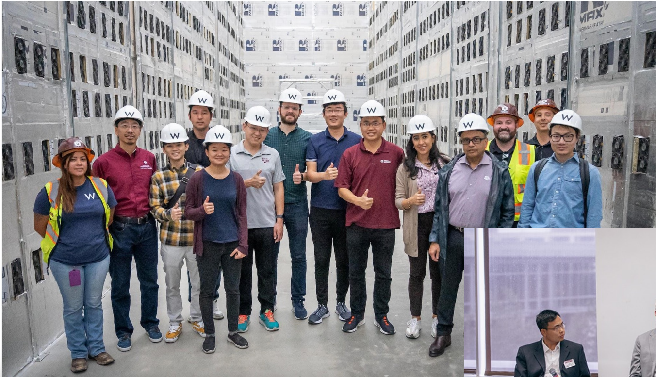
Site Visit to Riot (750MW)
